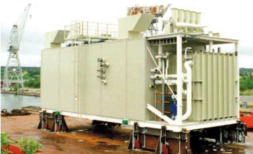
A 7 MW Hydraulic Power Unit, designed and built by Jotne. The unit generates electricity for a drilling rig.
