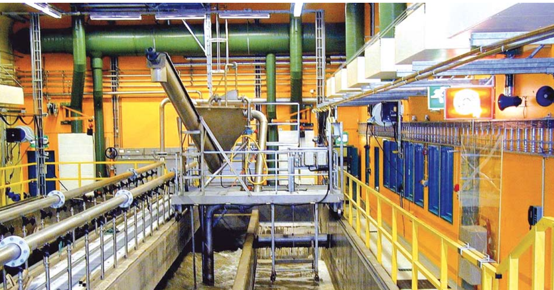
Waste water treatment plant
